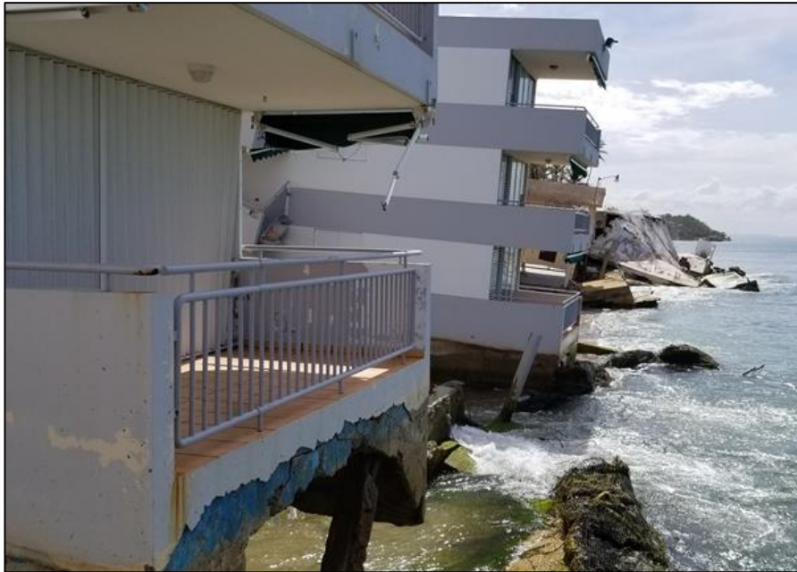
Hurricane Maria, 2017, Rincón, Puerto Rico
