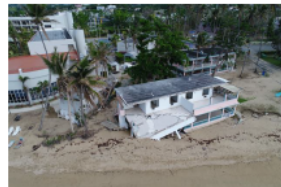
Figure 1. Failure of structure subject to surge, waves, and erosion.
