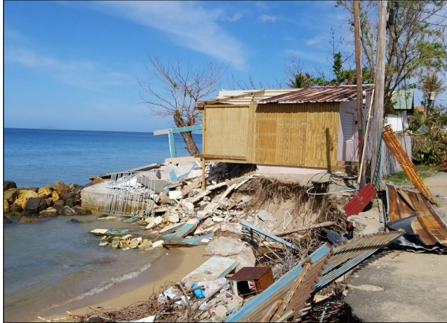
Hurricane Maria, 2017, Rincón, Puerto Rico
